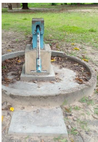
Photo : Protected well with broken hand-pump in Namala 2
