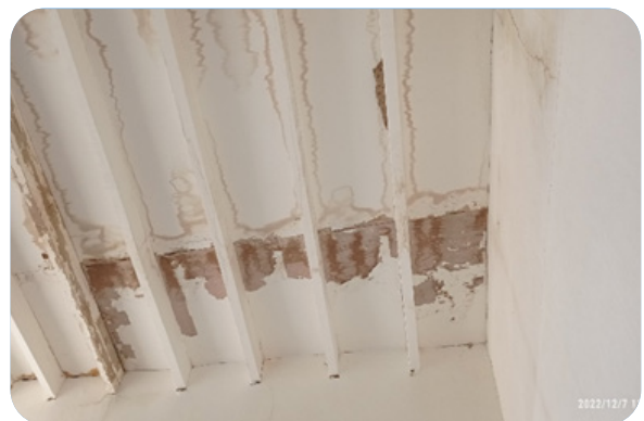
Figure 6 the hospital roofs conditions
