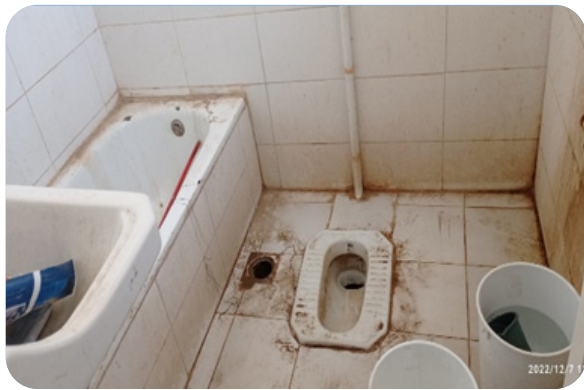
Figure 3 the bathrooms of the hospital conditions
