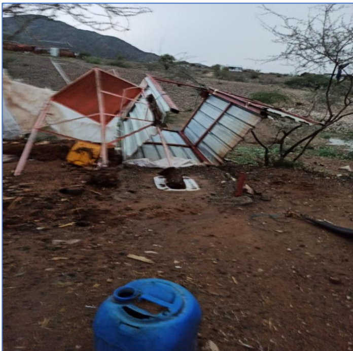
Photo 7 Damaged IDP latrine by the floods and strong wind- Al Dabayah IDPs site – Sep 04, 2022
