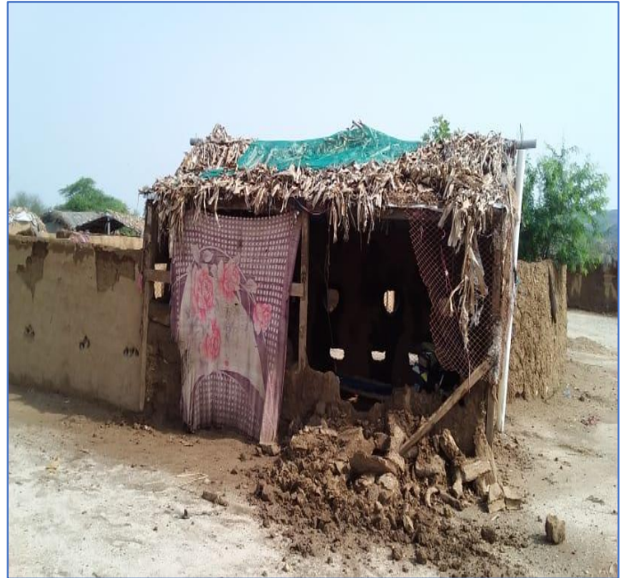
Photo 10 Shelter walls of mud collapse because of heavy rain and it need to be rehabilitated - Almebsham IDPs site – Sep 03, 2022
