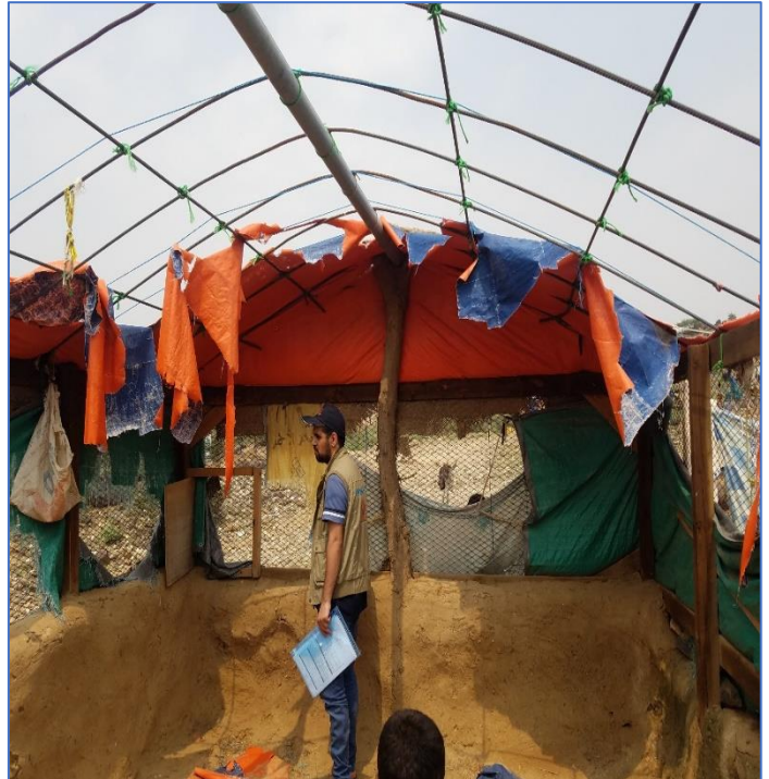
Photo 22 Partially damaged shelter - Alqafrah IDPs site - Sep 05, 2022
