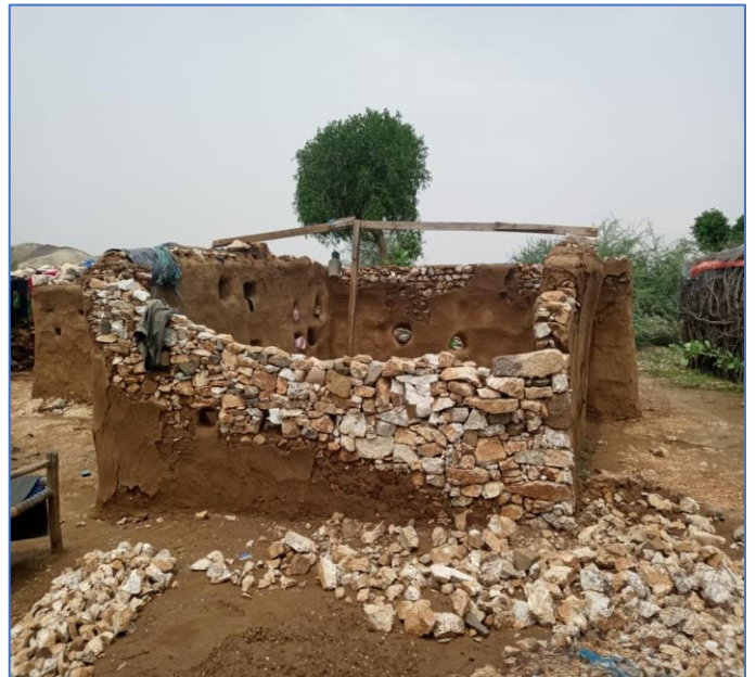
Photo 24 Damaged shelter by heavy rain - Malakh IDPs site – Sep 04, 2022
