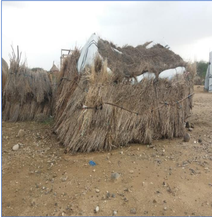
Photo 17 Destroyed Shelter by strong wind - Al Malab IDPs site – Sep 05, 2022
