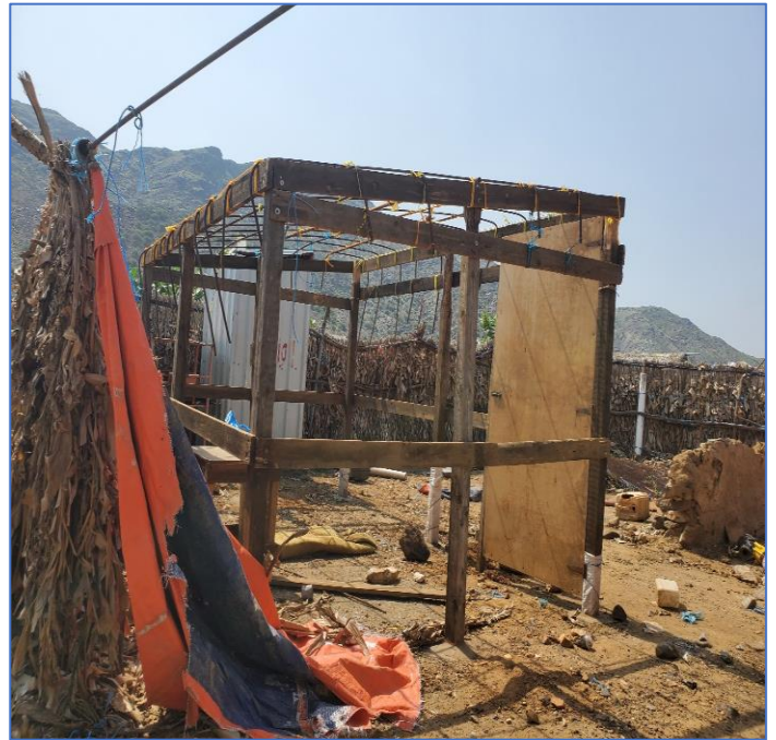
Photo 6 Partilly damaged shelter by heavy rain and strong wind - Al Dabayah IDPs site - Sep 04, 2022
