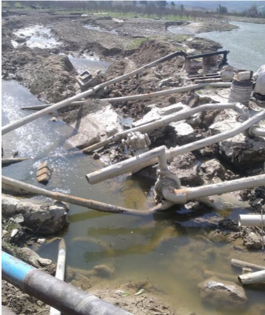
Damaged pipes, March 2023. ©FAO.
