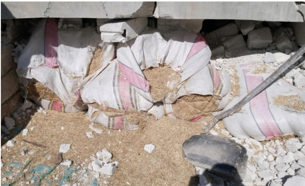
Damage to feed warehouses and storage, March 2023. ©FAO.
