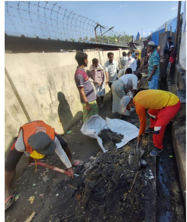
Old waste in drains
