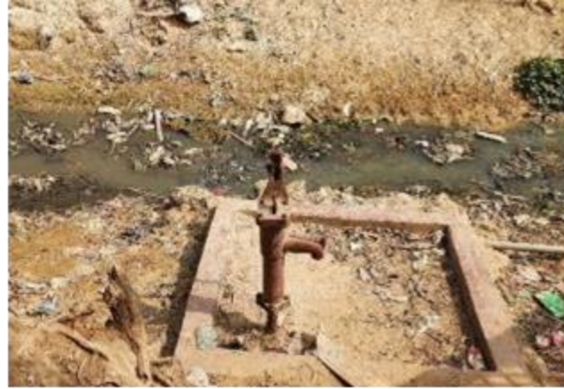
Tube-well on the Streambed
