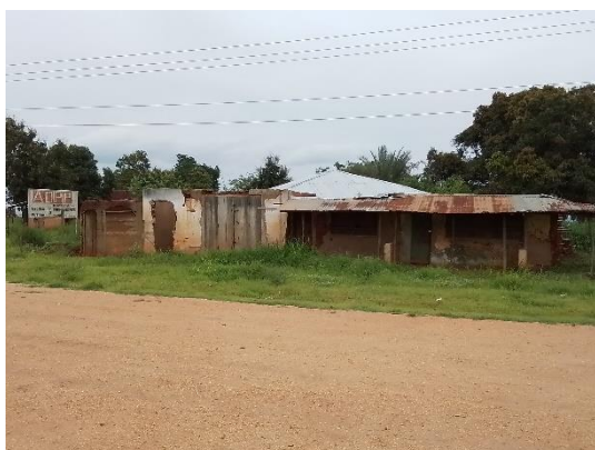
Figure 6- Commercial establishments destroyed
