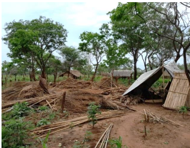
Figure 3- Shelter built with local materials damaged by rain
